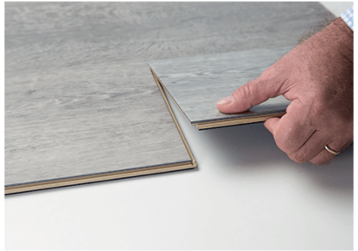
Slide the plank until it reaches the short side of the next plank.
